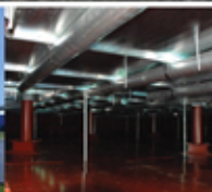
Internal Floating Roof
